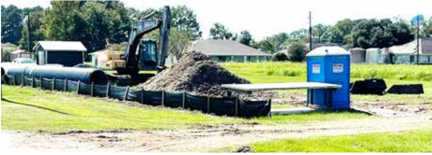
Pipes and equipment for the Ridgewood area drainage project.
